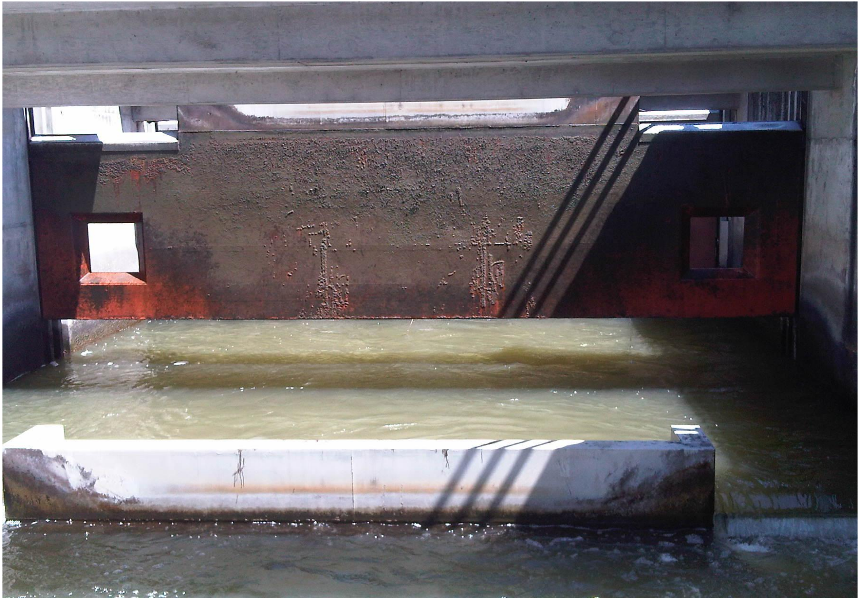
155 weir pulled at low forebay level. Exit weirs 154 - 159 condition being assessed for future rehab work.
